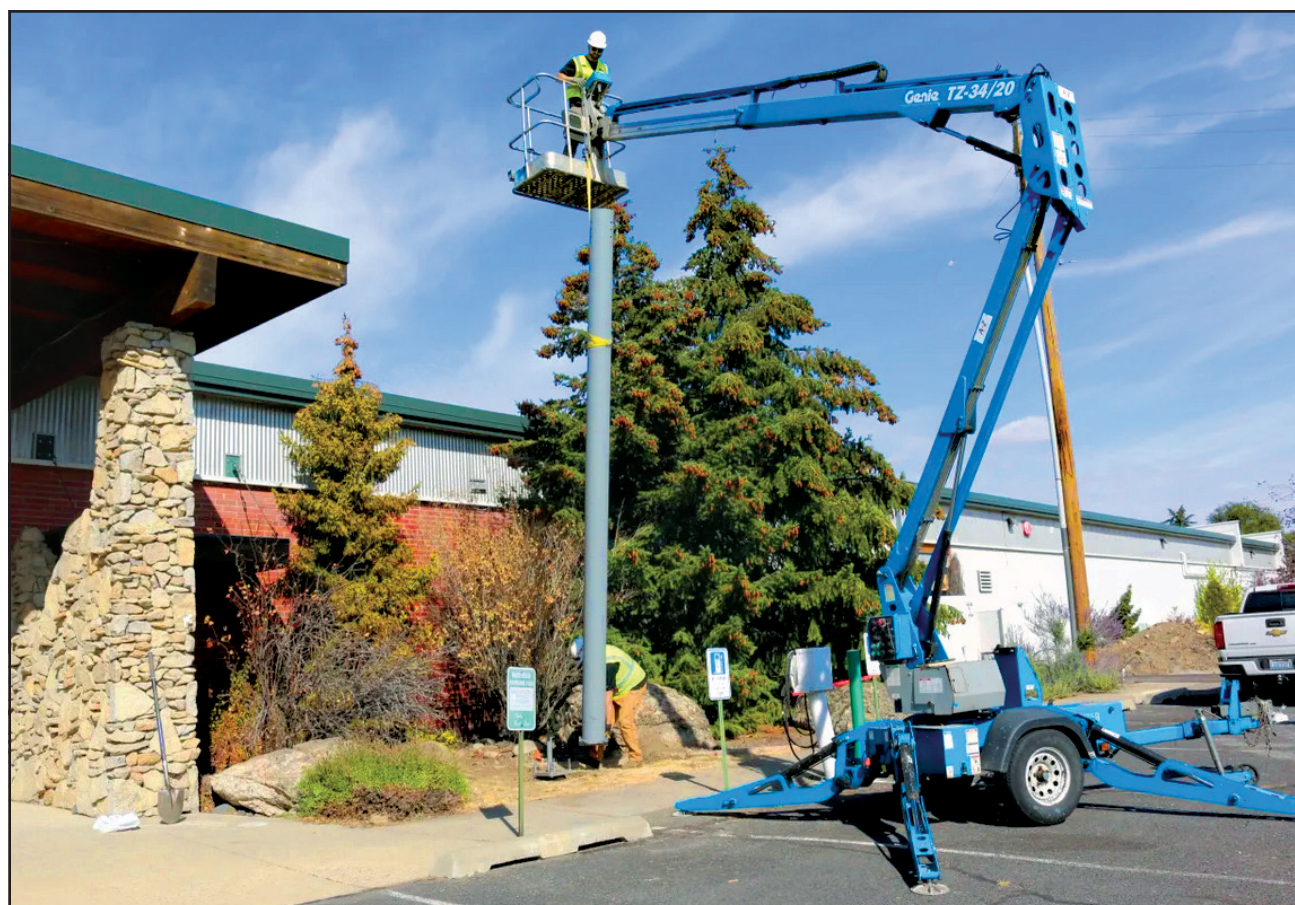
Fifty-foot-tall, small-scale cell towers such as this one could be critical to providing reliable, readily accessible cell phone service to underserved areas in rural Vermont. Strategically placed, the relay towers can significantly impact the “shadowing” effects of Vermont’s mountains and forests that cause cell phone signals to drop or be inaccessible in many rural settings. Courtesy of Easy Street Systems
